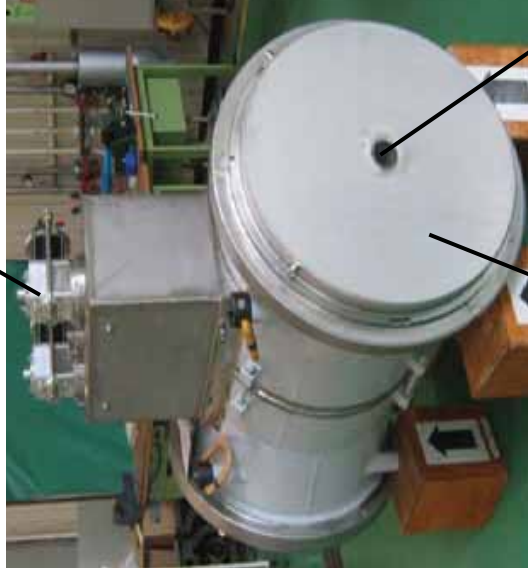
Refrigerators directly cooling SCM
